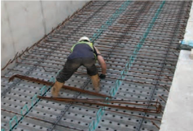
Panels sealed to support wall and abutting panel, then steel reinforcement positioned.
