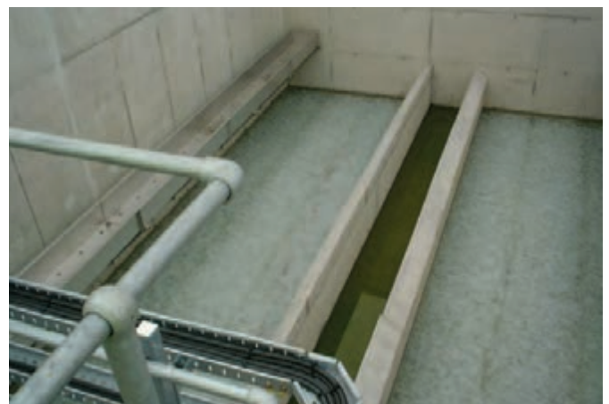
Air scour pattern test of finished filter floor (To prove level within tolerance).
