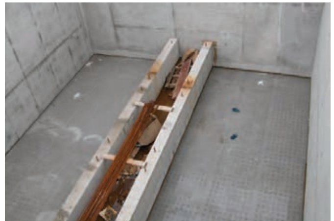
Concrete shortly after curing.
